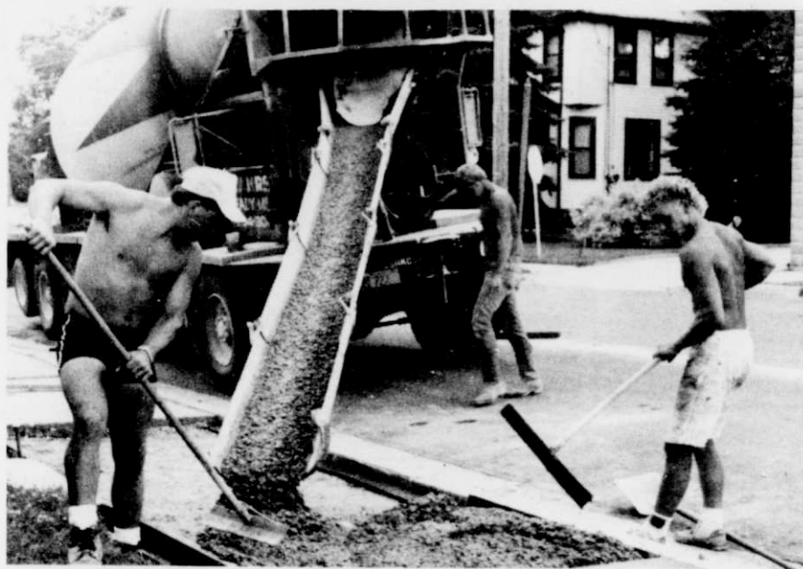
Sidewalk cracks in the village are now at a minimum as new sidewalks and repair has been going full speed ahead by the workers from Quality Concrete of Manawa. Pictured are the men pouring cement and laying out sidewalk on Parkview Drive.
