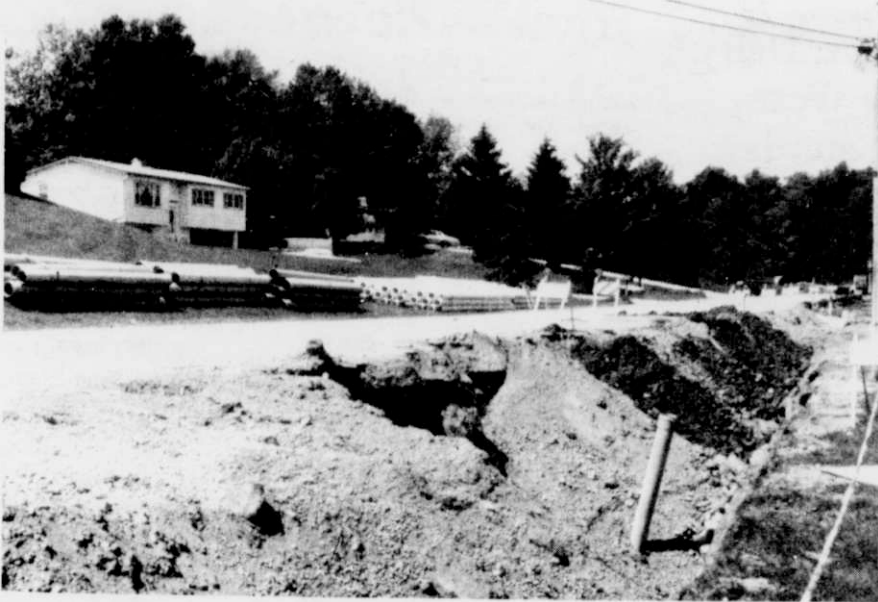
Work has begun on the installation of sewer and water services to residents along Bonnie Lane, which were annexed to the village last year. The work is expected to be completed by August 15th.
