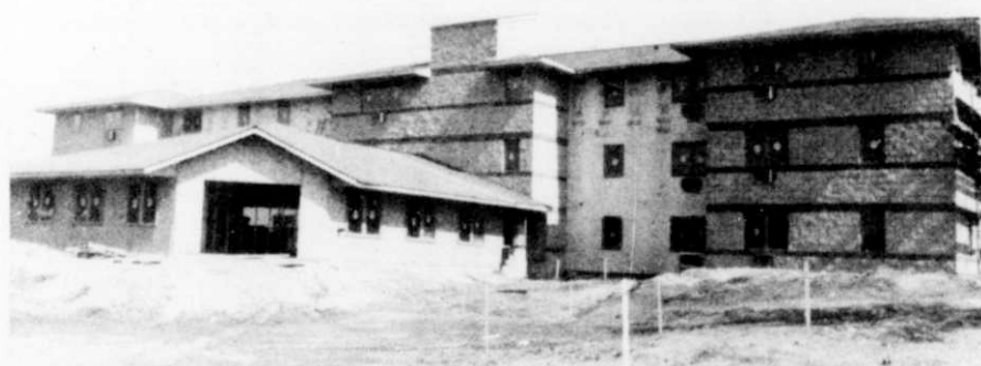
Mapledale Manor, Kewaskum, the elderly and CBRF project of Drs. Cesar and Aurora Sison is still under construction. The building is expected to be finished by mid-July.
