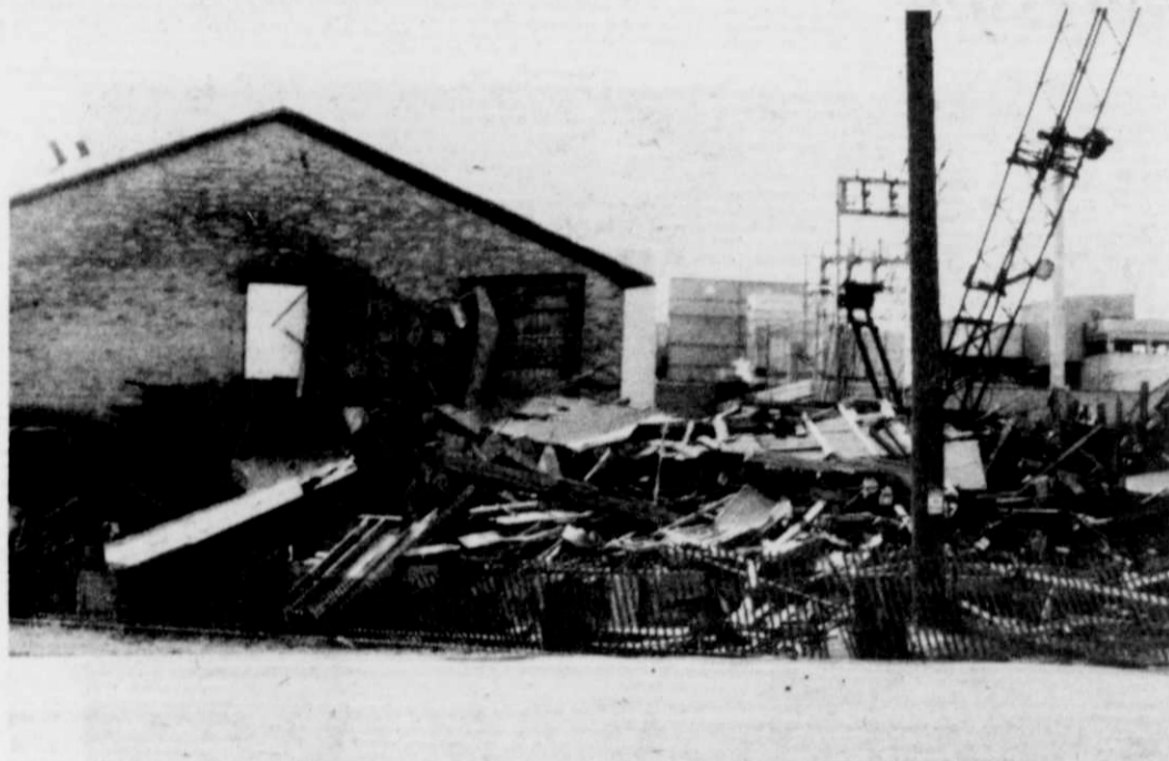
Pile of rubble after part of the Kewaskum Mill was recently torn down.
