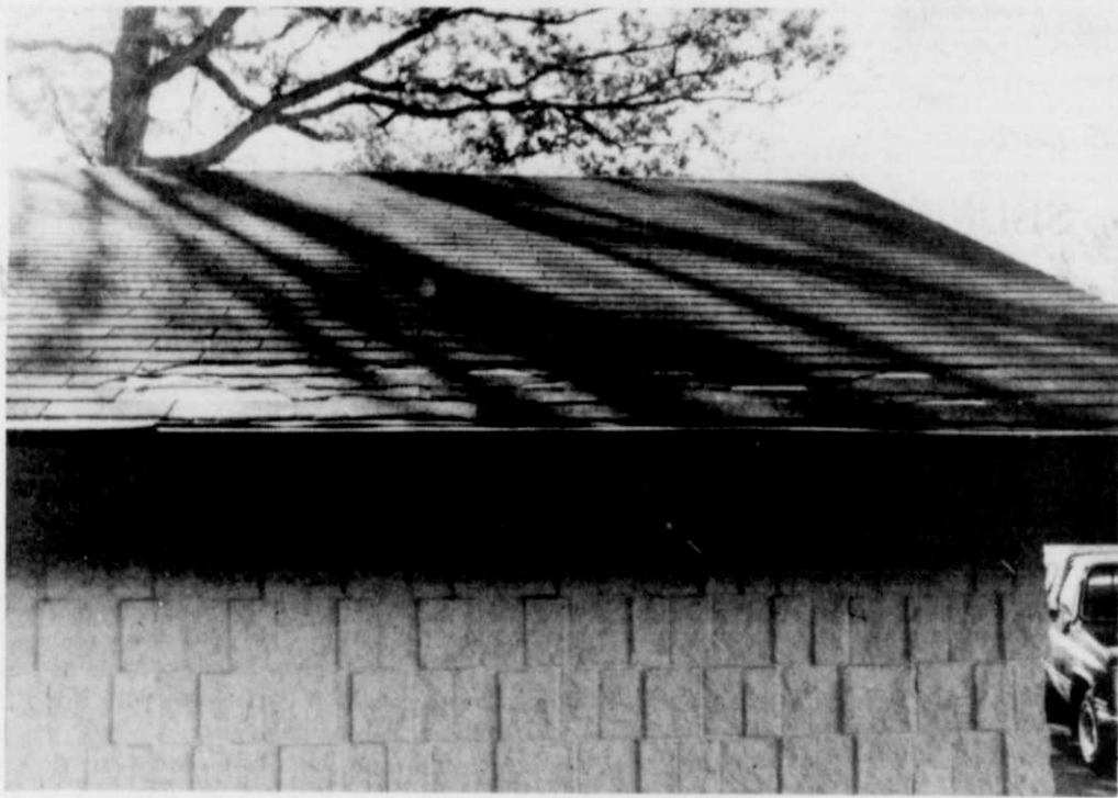
A section of roof shingles was torn off the shelter by vandals over the weekend.
