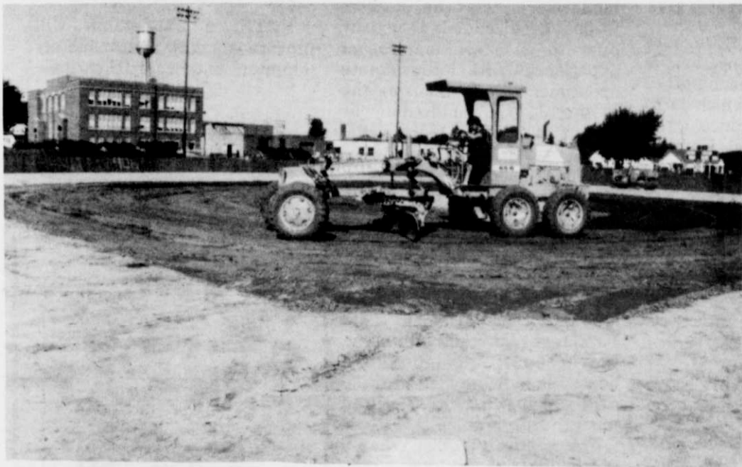
BALL DIAMOND REPAIRED... Work was begun on the high school baseball diamond to repair the infield and grass areas.
