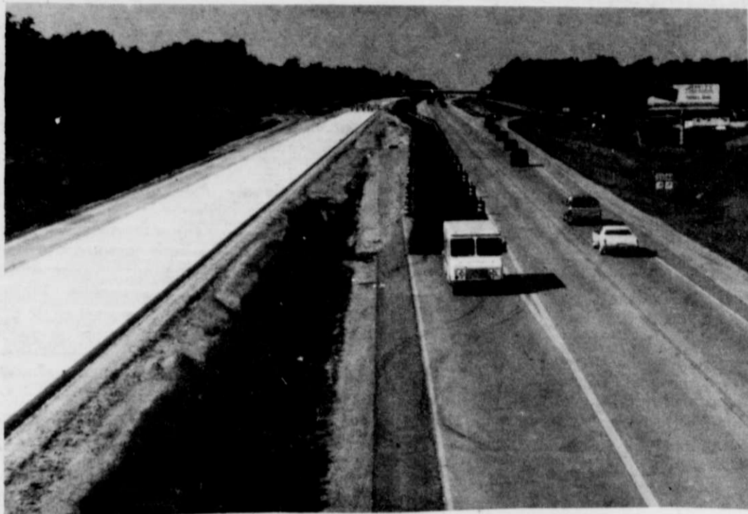
Construction of the Highway 45 bypass is progressing with paving of the two southbound lanes nearly completed. Work on the northern end of the bypass and on-off ramps has been. This view, looking north towards the Highway 33 intersection shows the northbound lanes which are handling the two-way traffic and the new southbound lanes.
