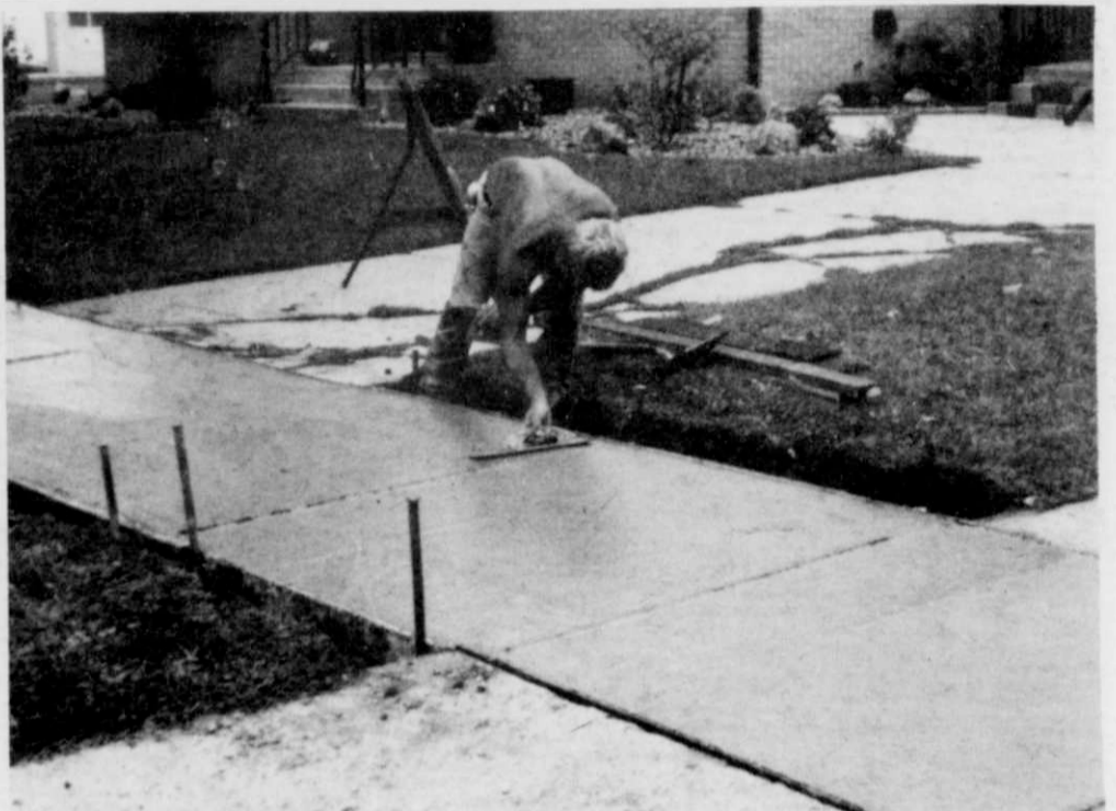
Here a worker applies the finishing touches to a brand new sidewalk.
