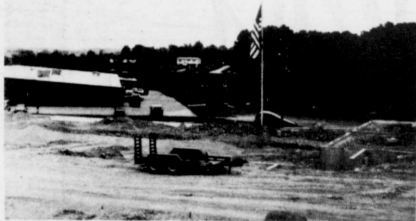
Preliminary work has begun on a 24-unit apartment complex being built by Tom Timblin of Kewaskum. The building will be erected north of the Kewaskum Shopping Mall, behind KL Home and Hardware.
