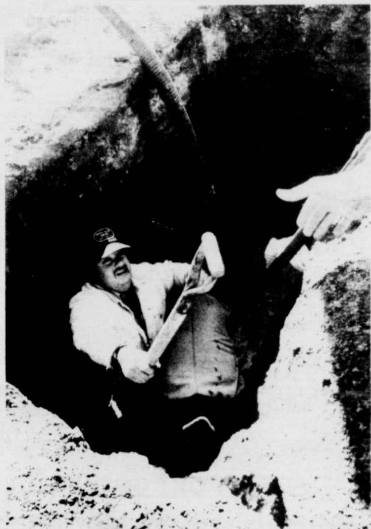
Public Works employee Alan Kuehl and Superintendent Augie Bilgo (bending over) spent several cold, wet hours repairing the broken main.
