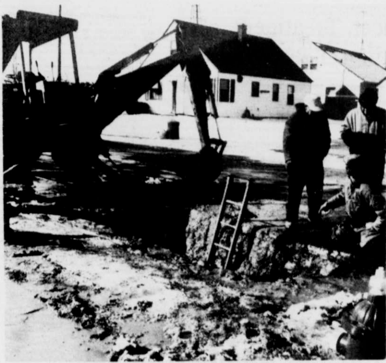
Public Works employees dug open the road to get at a broken water main near Bilgo and Third Streets. The break in the 8" main caused cancellation of classes at the high school Monday.
