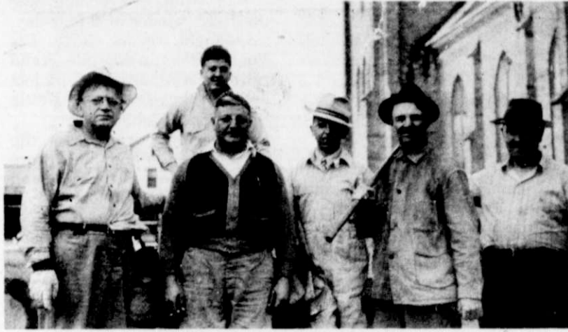
This is a photo of a work party at Holy Trinity Church in the early 1940's, removing stones, bricks and ground from the church basement to make way for the hall and kitchen. First row, left to right: Pete Haug, Norbert Becker, Pat Miller, Jake Harter and Joe Mayer. Back row: Joe Miller.
