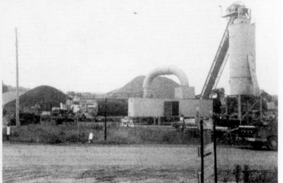
The portable asphalt plant set up on Highway 28 and Kettle Moraine stands like a giant metal redwood tree among the pines of the Kettle Moraine. Once the project is completed, the plant will be torn down and moved. The site is already being graded and prepared for seeding to return it to its original state.
