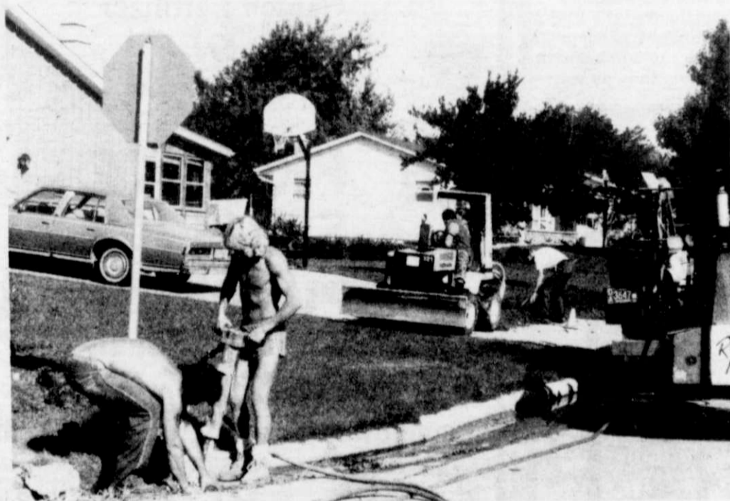
Village and construction crews worked on removing old curbing and preparation beds for the installation of sidewalks along Brooklane and Clinton.
