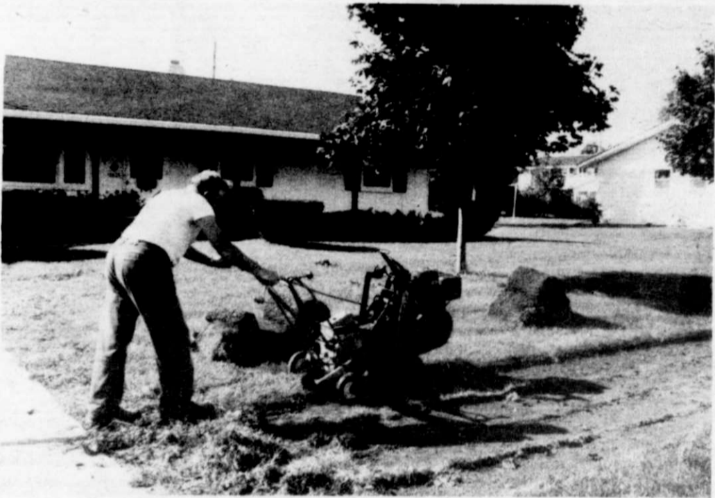
Butch Bauer cut and removed sod along Brooklane in preparation for the laying of sidewalks.
