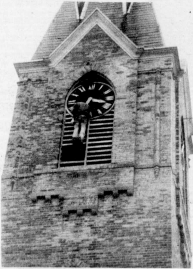
PAINTING THE CLOCK — Work was completed on the face of Holy Trinity Church clock during the recent remodeling and redecorating project of the church. Note the precarious position of the painter standing on a plank which extended from the inside of the steeple. All is in readiness for the 125th Anniversary celebration of the church which will be held Sunday, May 25. (See front page item).
