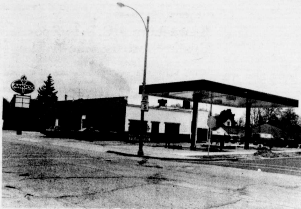
Bob Kohn's new Amoco quick stop mart and self-service gas station is taking shape.
