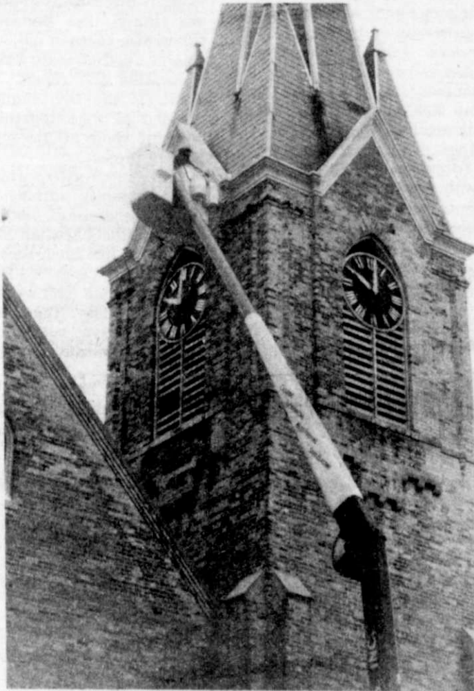
A Holton Brothers employee works on replacing mortar on one of Holy Trinity's steeples.
