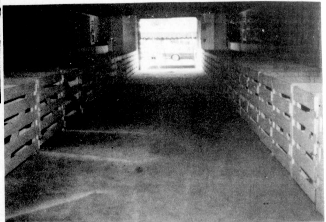
A picture of the finished project. This picture was taken a few days before county fair was to begin. The work proved to be worthwhile as less people walking through the barn got wet feet.
