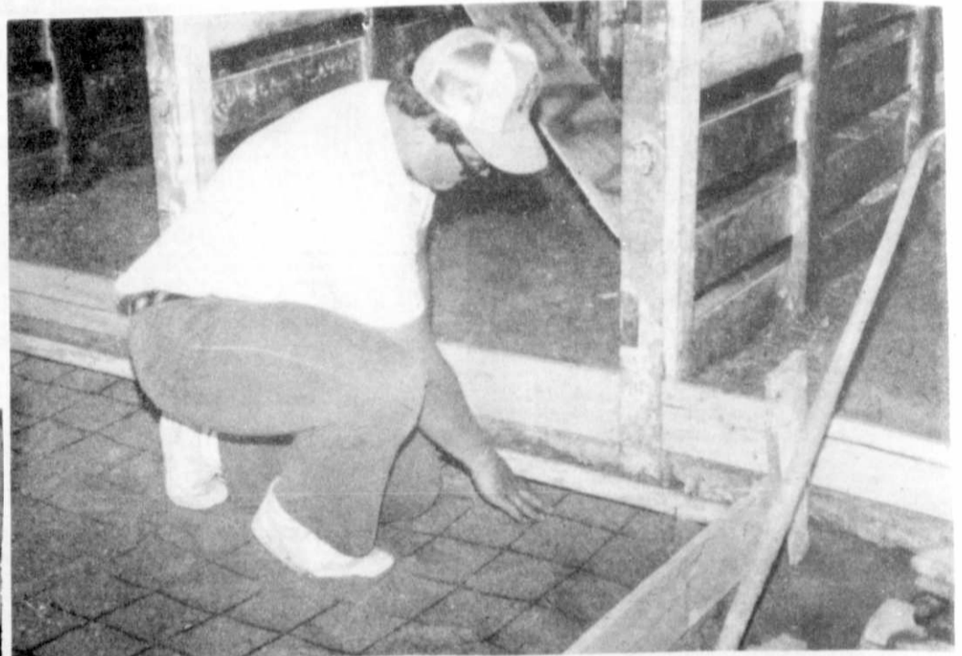
Joel Junk helps lay pipe on both sides of the aisle for leveling the cement. A vibrator with an engine was used to level off the cement.
