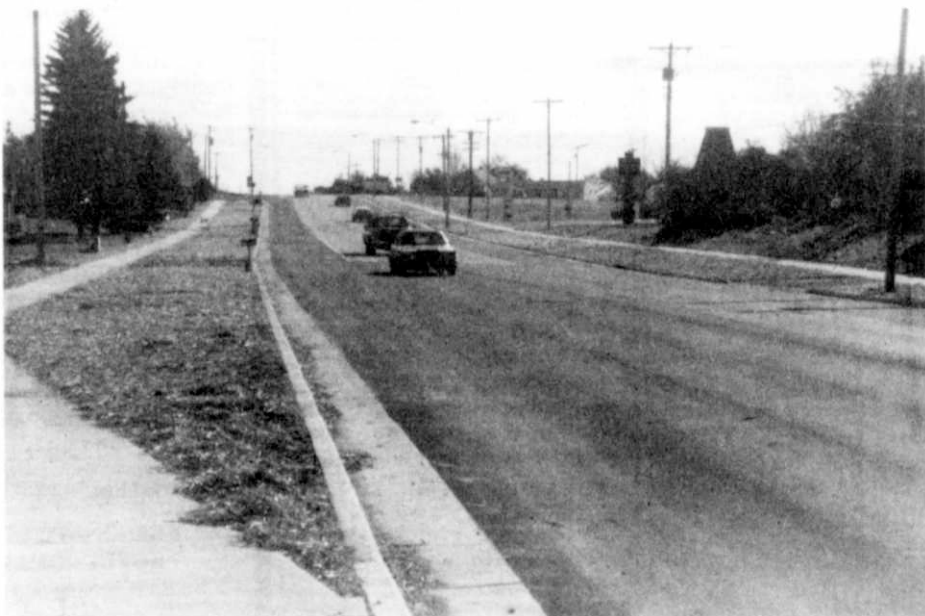
FINISHED AT LAST — The final work in completion of Kewaskum's TIF District new sidewalk, curb and gutter and road widening project along Highways H and 45 was the landscaping, seeding and covering new grass seed. The project was finished last weekend. Looking south on Hwy. 45 toward H, the sidewalk extends to the end of the homes almost to the former Hydraulic Gear, Inc. on the east side of the road and to Prospect Dr. near Roger and Dan's Auto Service past the Kewaskum Mall on the west side. On Hwy. H west, the sidewalk extends past Bel-Ric Dr. and the apartment buildings almost to the creek on the south side and just past Milan Dr. on the north side. On the north the sidewalk begins in the area of the Kewaskum Fire Department station on Fond du Lac Ave.
