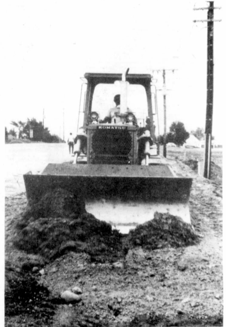
CONSTRUCTION UNDERWAY — Work is now underway on the reconstruction of the roadway and installation of curbs and sidewalks along 29 properties on Highways 45 and H on the south end of the village. The work is being done by A. R. Melichar Concrete Contractors. Chuck Voge photo
