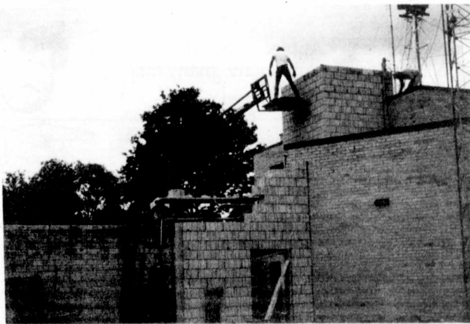
Work is moving right along on the addition to and remodeling of the Kewaskum Municipal Building.
