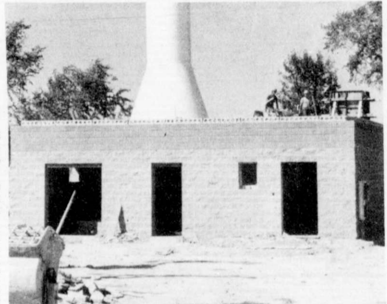
THE NEW PUMP HOUSE for Kewaskum well #3 is beginning to take shape. Workers were doing cement work on the building's roof area. The tower for well #3 can be seen in the background.
