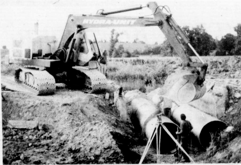
HWY. 28 PROJECT — Work is progressing on the reconstruction of State Trunk Hwy. 28 from U.S. 41 to Kewaskum, which began in spring. Shown is the installation of culverts close to Mullen Road at the Joe Schmitt and Jim Maul farms. (Claire Ciha Photos)
