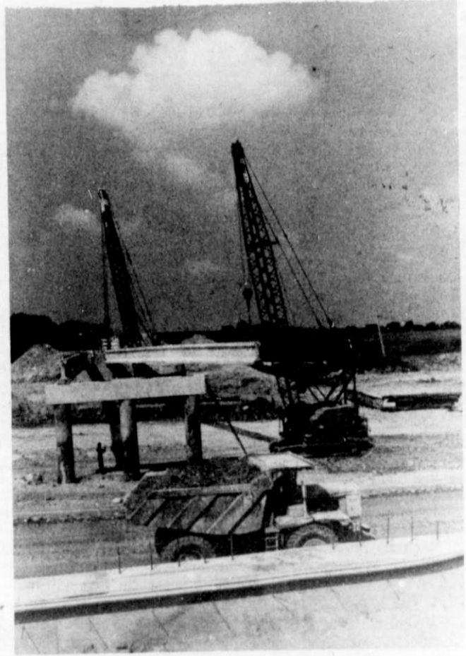
Crews and cranes lift a concrete bridge support span into place. The new bridge will eventually carry Western Avenue traffic over the Highway 45 bypass. Western Avenue is located between the 41-45 junction and Jackson. Staff photos by Gerry Mueller
