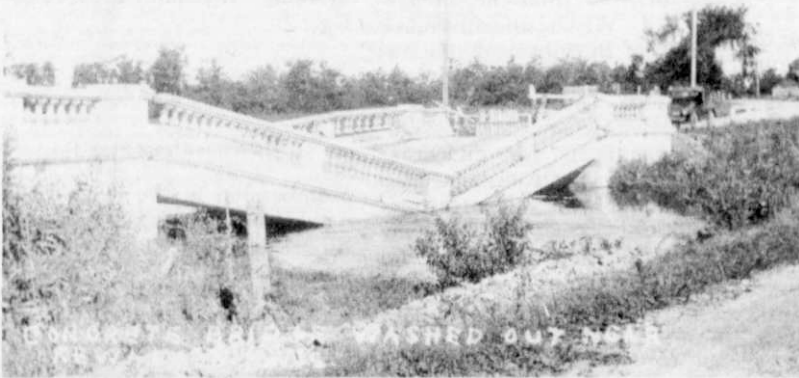
Fellenz bridge collapsed at the Fond du Lac-Washington County line north of Kewaskum. Water was 15 feet deep.
