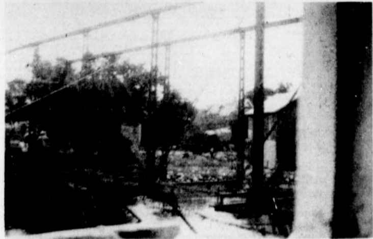
These two photos show the dismantling of the old steel bridge across the Milwaukee River on lower Main Street in Kewaskum. The bridge was dismantled about 1928 or 1929.
