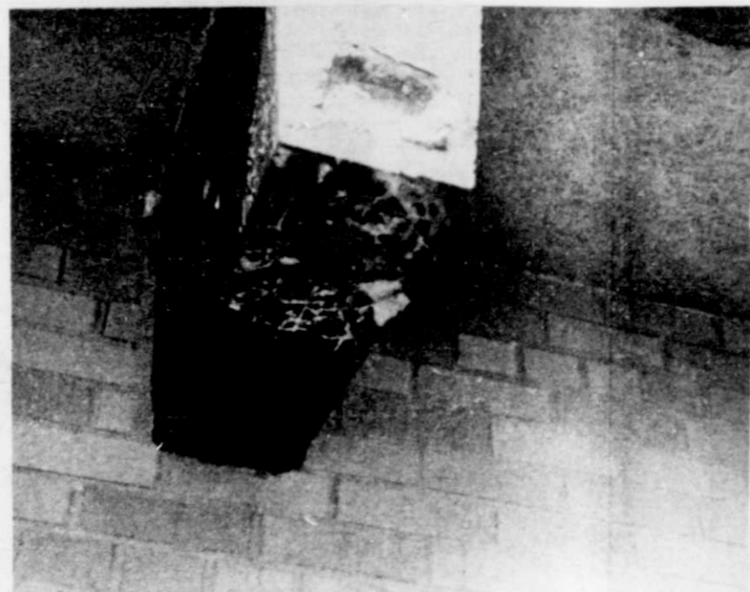
Wayne Elementary — Water damage on steel and concrete roof beams.
