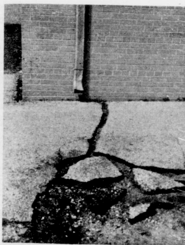
Beechwood Elementary — Rain water runoff damage to blacktop area.
