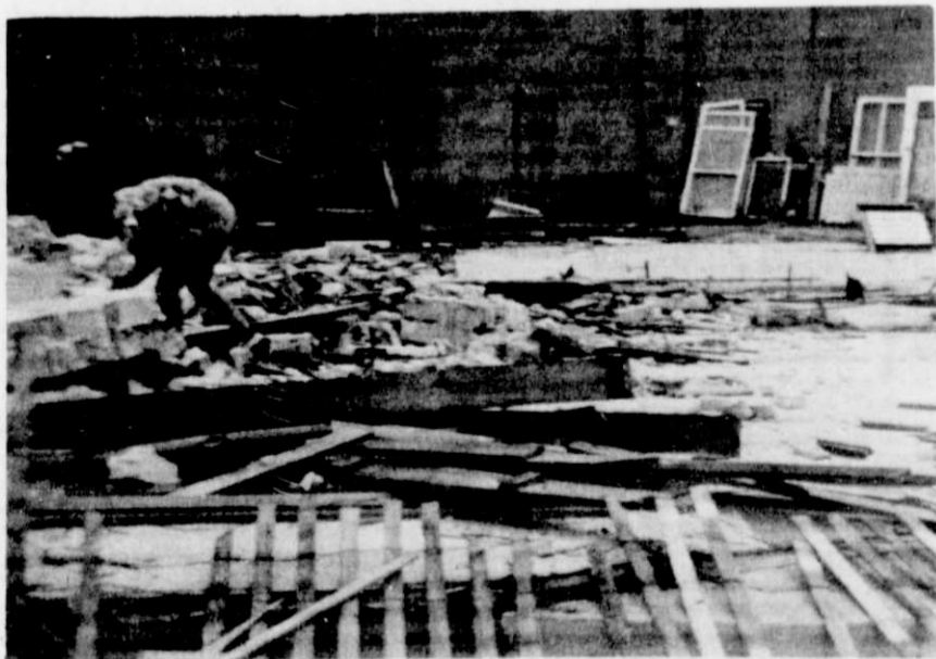
The building completely razed.
