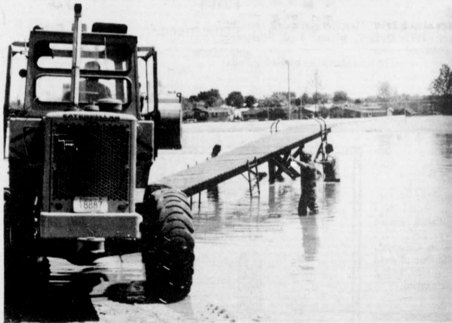
"Crickets" backing the pier into the pond. Augie [left], "Schmitt" and "Mooch" working on anchoring the mobile pier.
