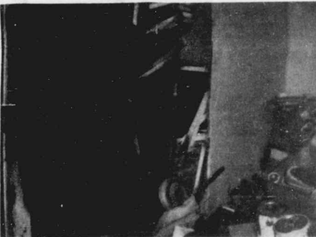
Wall and stairs where fire apparently started.
