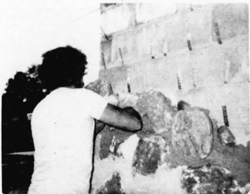
Marshal Reysen, member of the Kewaskum Historical Society, working on the foundation of the log house being erected on the site of the Historical Society on Park View Drive in Kewaskum. Marshal is proud to be working on the restoration of his forefathers' home. The Reysen family donated the log home to the Historical Society. It was dismantled and will again be assembled to its original structure on the new foundation. All donations from the Early Farm Days held recently and any other donations will be used in the reconstruction of the log home.
