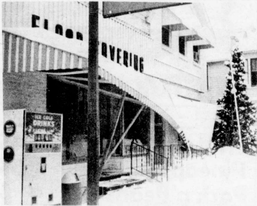
CANOPY COLLAPSES — The canopy in front of the K & R Carpeting Store on Main Street collapsed over the weekend from the weight of the snow. Many village residents were seen cleaning off the snow from canopies and roofs this week.
