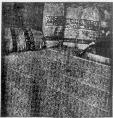
-O-PAK Insulation spread between the joists under an attic floor.
