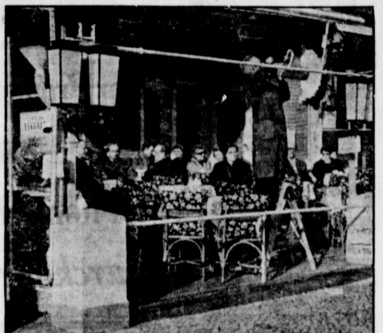
TAKES THE CHILL OFF COFFEE —Patrons of this West Berlin sidewalk cafe can now enjoy their coffee out-of-doors, regardless of the weather. Workman, center, is installing an infrared heating unit for his customers' comfort. Glass screens at left and right cut off chilling drafts.
