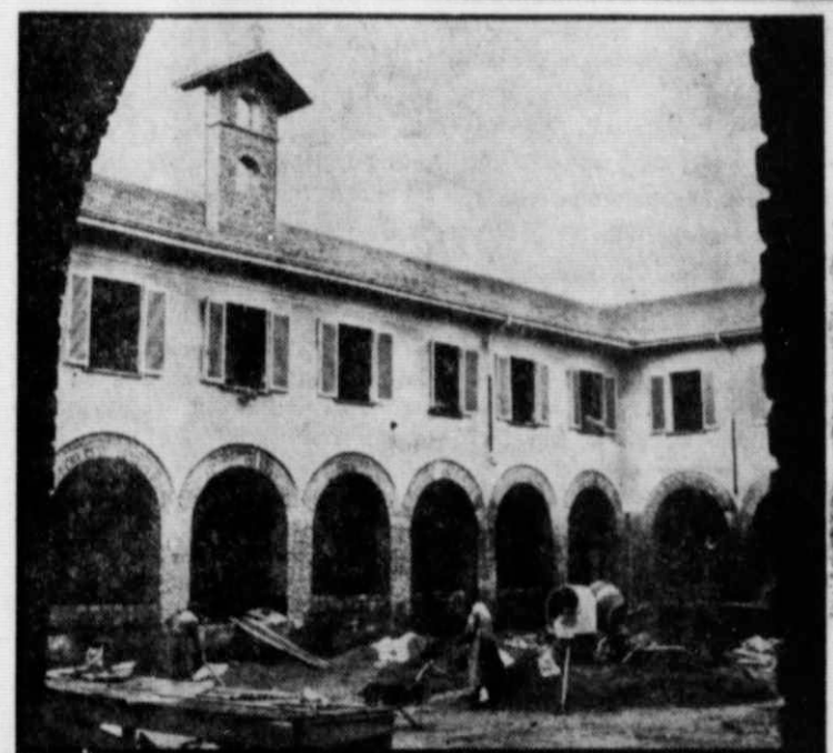
NUNS BUILD OWN CONVENT —A group of nuns and volunteer workers bend to the task of completing a convent near Turin, Italy. After taking lessons from masons for two months, the Carmelite nuns began work on the project, money for which was donated by local parishioners. When the convent is completed, the nuns will retire to a life of cloistered silence.
