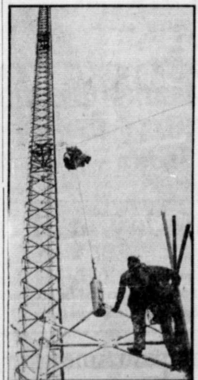
HIGH, CLEAR VOICE —Preparing for any possible complete severance of communications between Western Germany and West Berlin, workmen ascend a 150-foot very-high-frequency tower at Heckeshorn, in Western Germany, to prepare it for transmission. Heckeshorn station can route messages throughout Western Germany.
