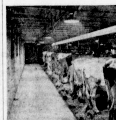
The above picture illustrates lighting outlets at 12-foot intervals on the center line of the litter alley and every 20 feet on the center line of the feed alley.
