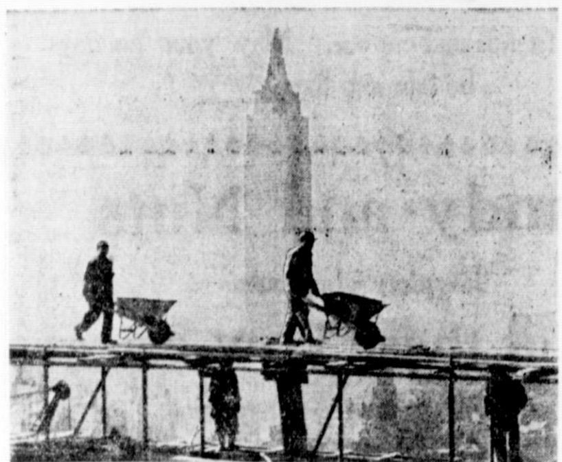
MONUMENT TO PEACE . . . This new view of progress being made in construction of the United Nations world headquarters in New York City shows workmen carting their wheelbarrows of cement on the 39th floor, in the shadow of New York's tallest skyscraper, the Empire State building.
