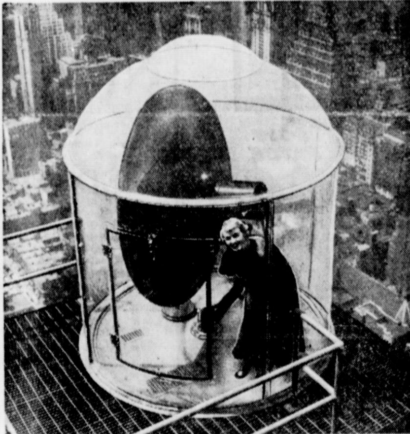
TOPS IN TELEVISION . . . Lodged on the pinnacle of New York's skyscraping RCA building, like a translucent bubble in the metropolitan air, is the new NBC television plexiglass radome housing receiving equipment for television. It's all-weather proof—cool in summer, warm in winter—as video star Kyle MacDonnell can attest after inspecting the "dish" which serves as a receiving antenna.
