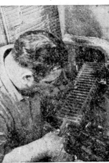
Picture shows final step in the converting process—replacement of the coal grates in the furnace.
